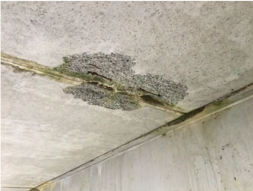
Damage to deck Panels 1 and 2 on right approach
