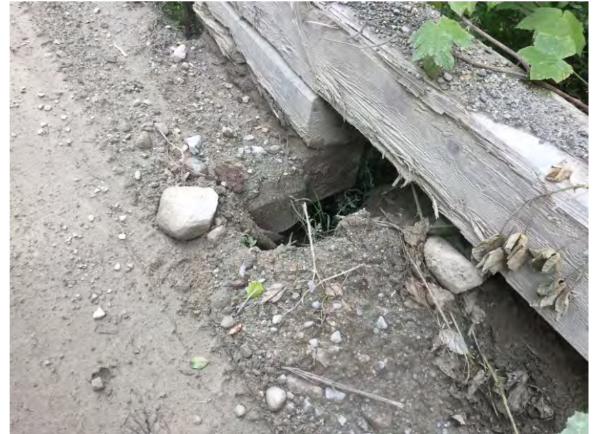
Failing fill at left upstream
