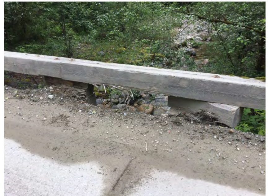
Rotting risers and blocks
